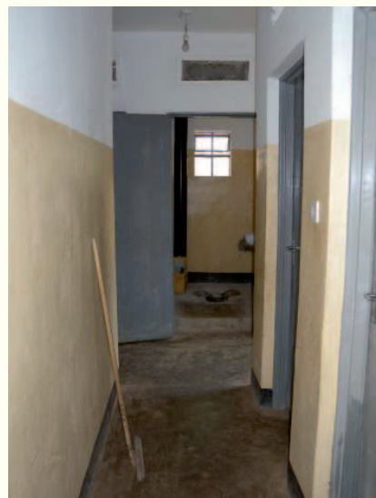
Picture 4: Indoor UDDT for hospital staff (Kitgum, Uganda).
