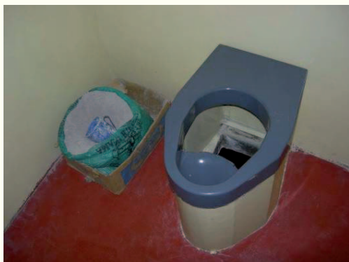
Picture 3: Sitting UDDT for an office building (Arua, Uganda).
