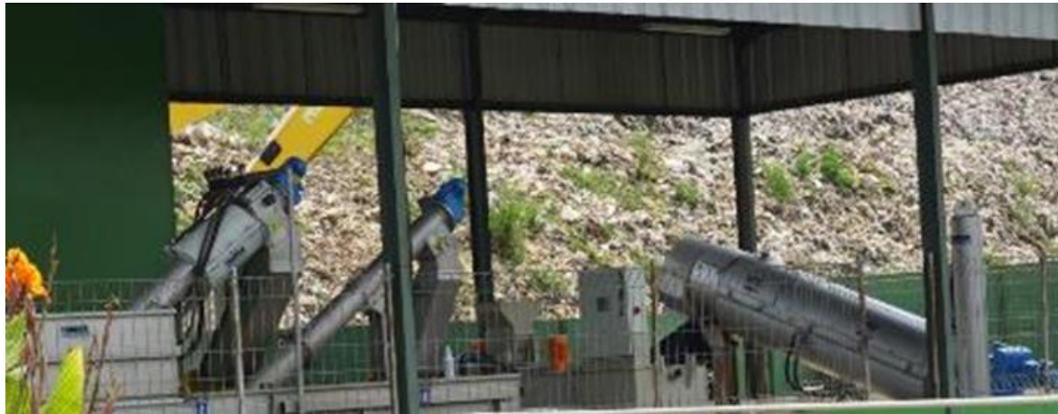
Figure 7.4: Mechanized decanting station using screw press technology in Bekasi City, Indonesia
