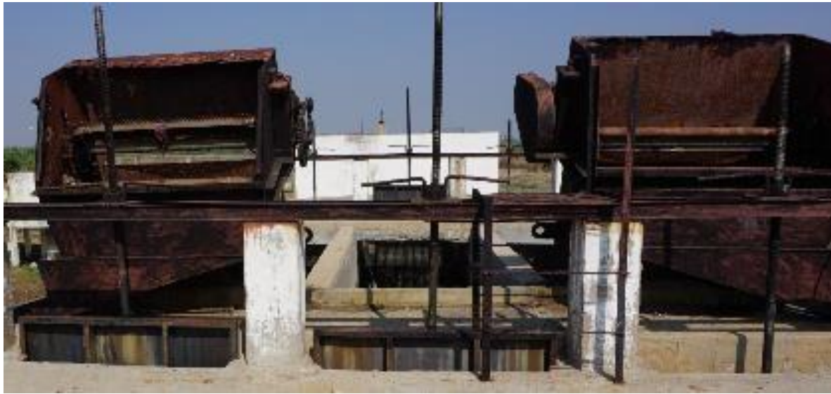
Figure 2.6: Screening system at head works
