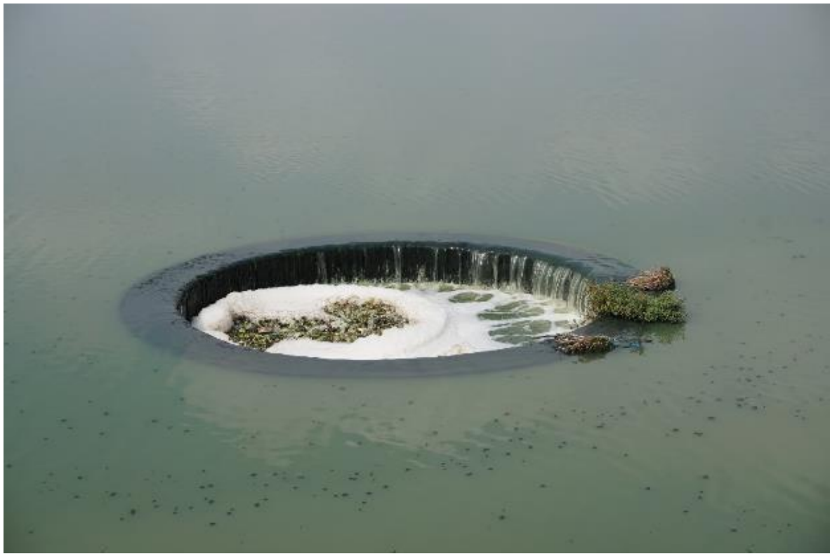
Figure 2.14: Facultative pond outlet structure
