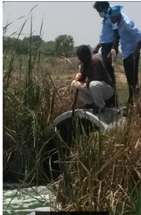
Figure 2.17: Discharge Pipe for Final Effluent
