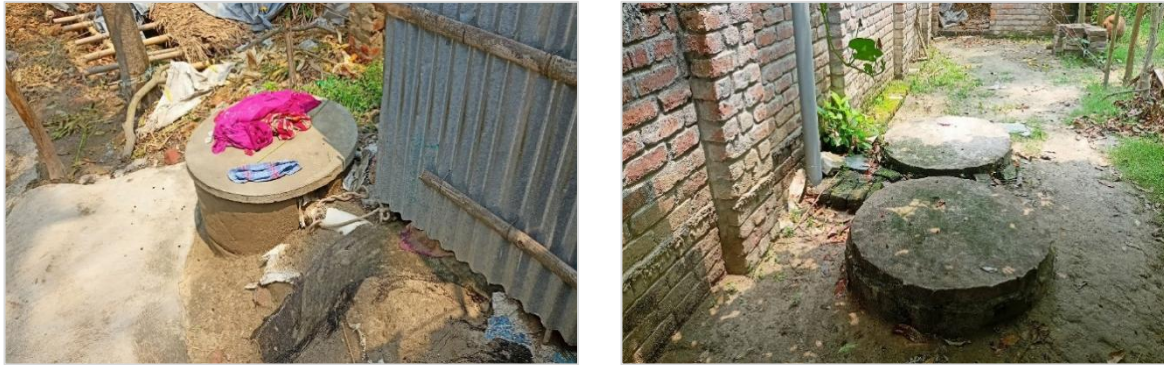
Figure 6: Containment technologies and their connections in Charghat Municipality (Source: Field Survey 2023/ O.CREEDS_WaterAid Bangladesh).
