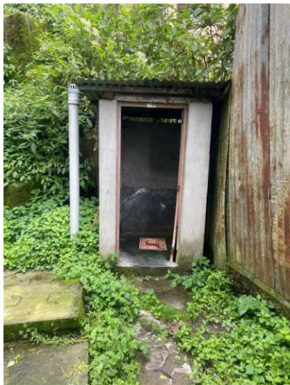
Figure 10: A toilet is connected to the septic tank with a gas vent outlet (Source: Sachin/NIUA/2024).
