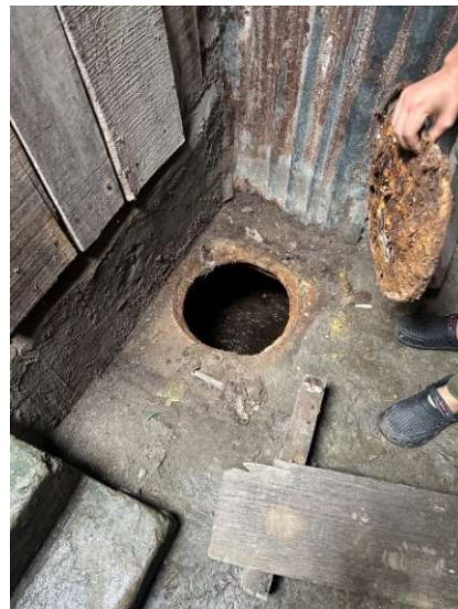
Figure 11: Lined tank (Source: Anant/NIUA/2024).
