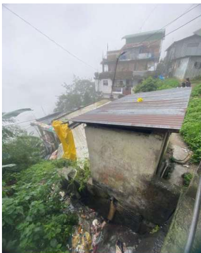
Figure 7: Toilet discharge into the open drain (Source: Sachin/NIUA/2024).
