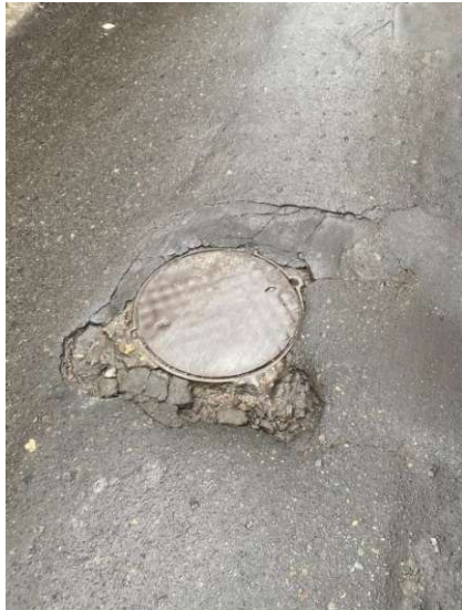
Figure 8: Sewer Line Manhole, Ward 11 (Source: Sachin/NIUA/2024).
