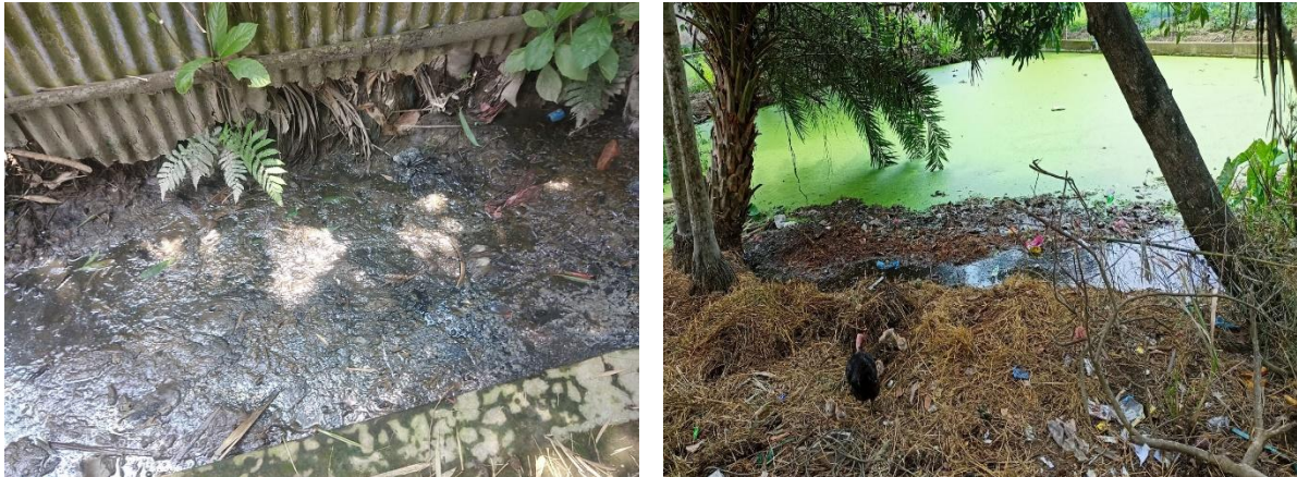
Figure 6: Containment technologies (single pit with direct connection with drain and waterbody) in Kamalganj Municipality. (Source: Field Survey 2023/ O.CREEDS_WaterAid Bangladesh).
